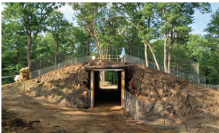
Tunnel jump and walk path through for spectators going to the peak of the track.
